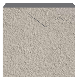
Irregular substrate (crazed and repaired)
